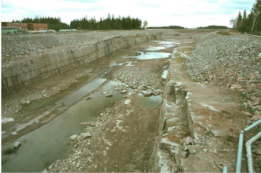
Figure 2-4. Sheet joints visible in the sides of the canal between the Baltic Sea and the nuclear power plant at Forsmark (Figure 5-14 in Follin 2008).
